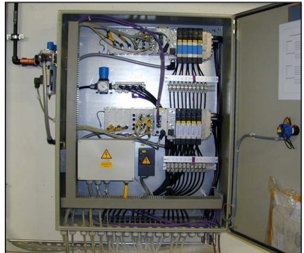
Figure 10: Control cabinet with valve terminal
