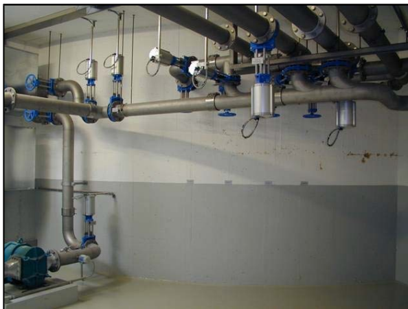
Figure 9: Pipe gallery in a wastewater treatment plant
