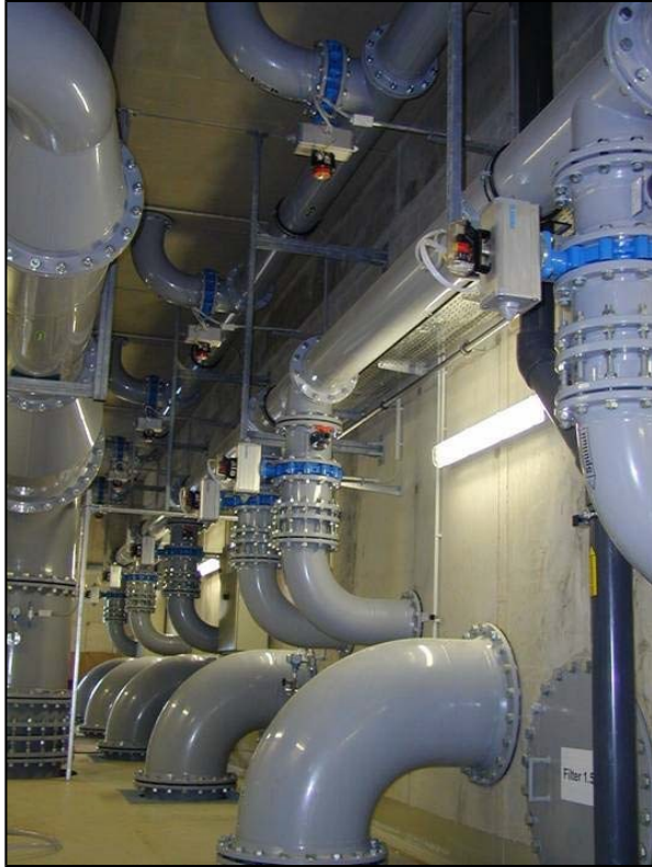
Figure 8: Pipe gallery in a water treatment system
