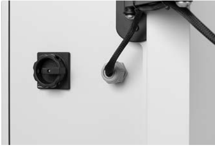
Figure 6. Main power switch.
