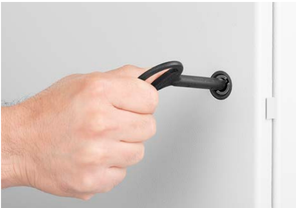
Figure 7. Locking the electrical panel door to prevent unauthorized access.
