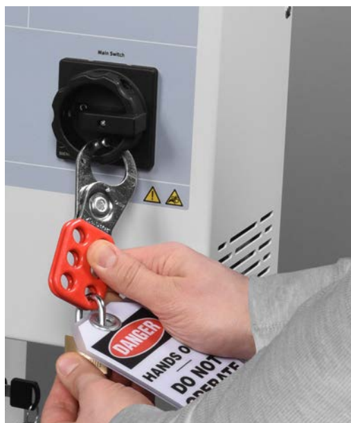
Figure 36: Lock-out/Tag-out device on an electrical switch.
