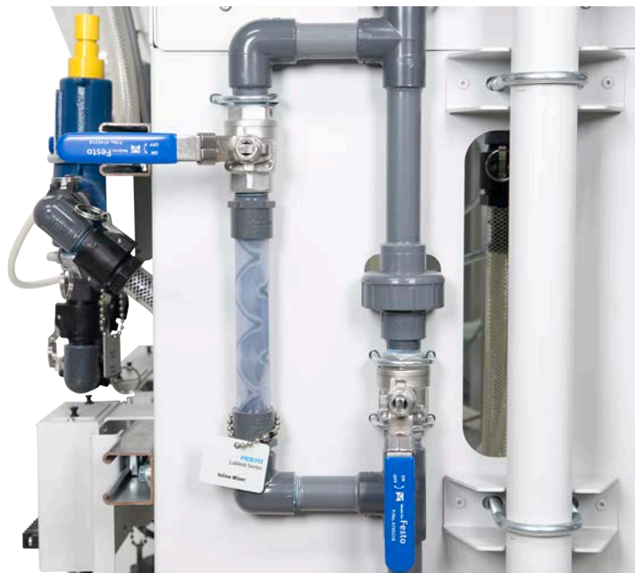
Figure 6: Inline mixer and pressure safety valve.
