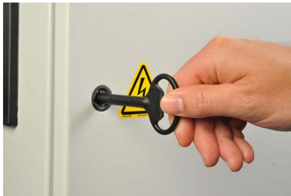
Figure 35: Lock the electrical panel door to prevent unauthorized access.
