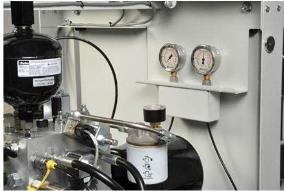
Figure 36: Pressure gauge guards.
