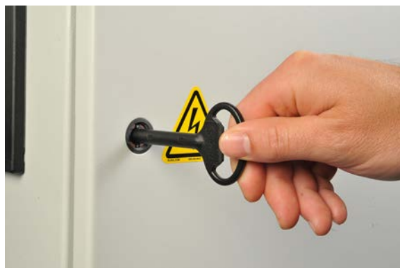
Figure 31: Lock the electrical panel door to prevent unauthorized access.
