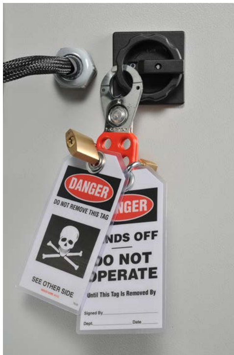
Figure 34: Installation of the lockout hasp, padlocks and tags.
