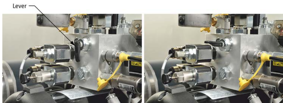
Figure 35: Depressurizing the hydraulic accumulator.
