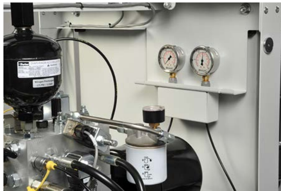
Figure 32: Pressure gauge guards.
