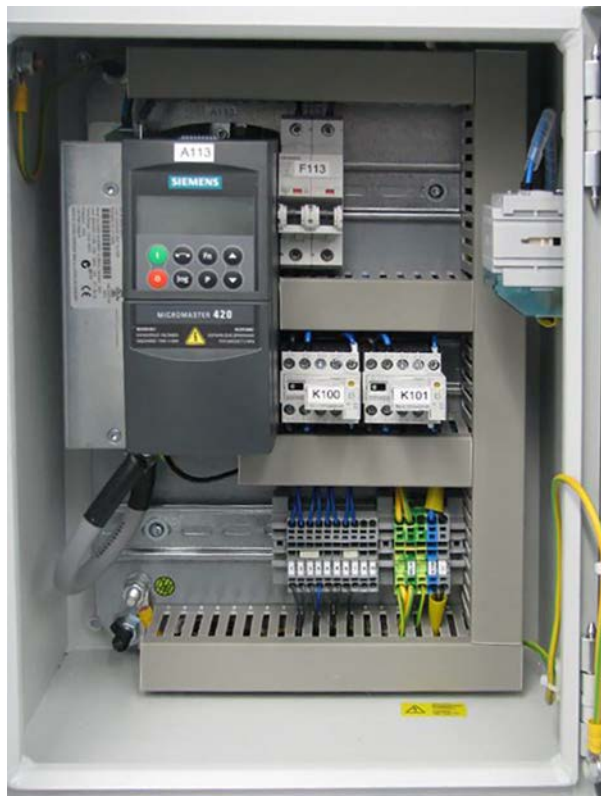
Figure 34: Electrical cabinet with frequency convertor.
