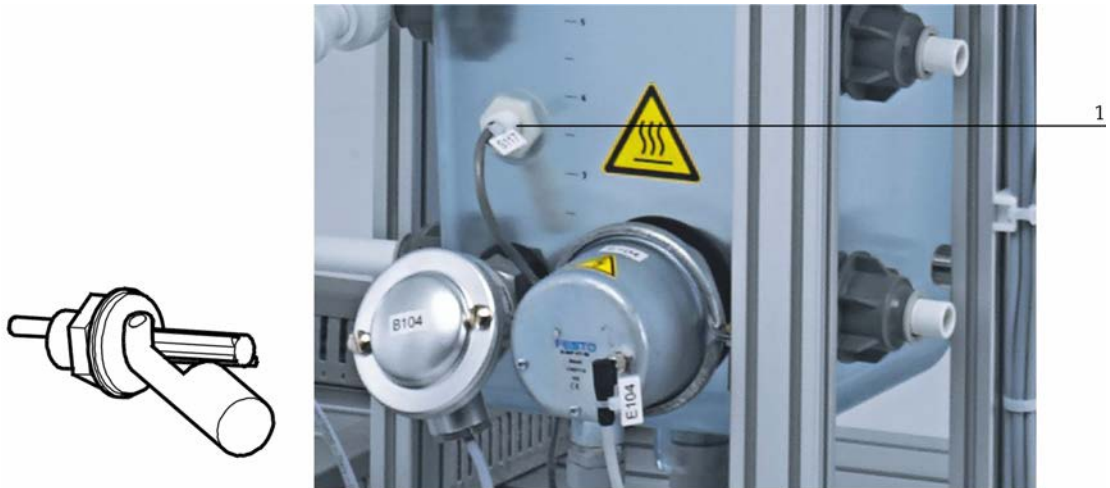
Figure 7: Float switch as switch-on protection for heating.
