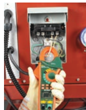
Maintenance and troubleshooting
