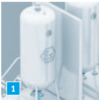
Inertisation of tanks and process equipment.
