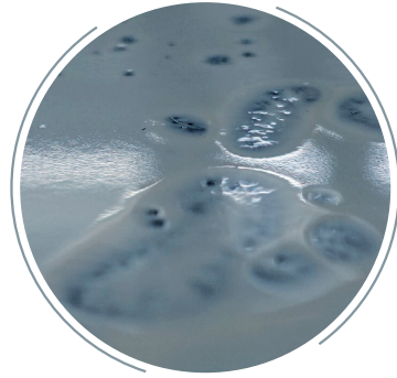
Paint defects – caused by paint-wetting impairment substances
