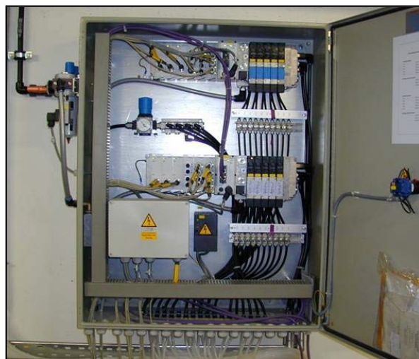
Figure 10: Control cabinet with valve terminal
