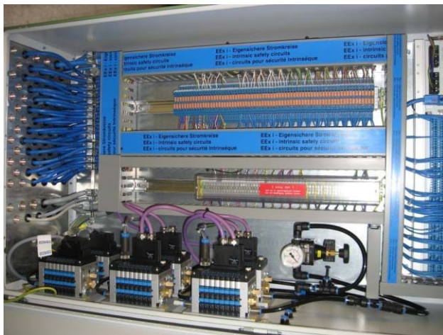
Figure 14: Valve terminal cabinet in ATEX zone 2 with valves for a safety instrumented system.
