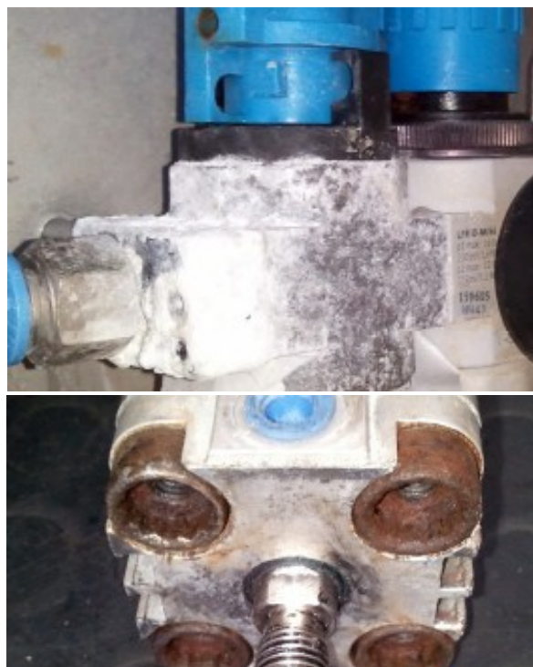
Incorrect choice of materials – typical damage profiles
