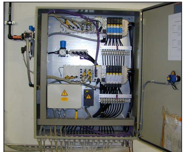
Figure 10: Control cabinet with valve terminal
