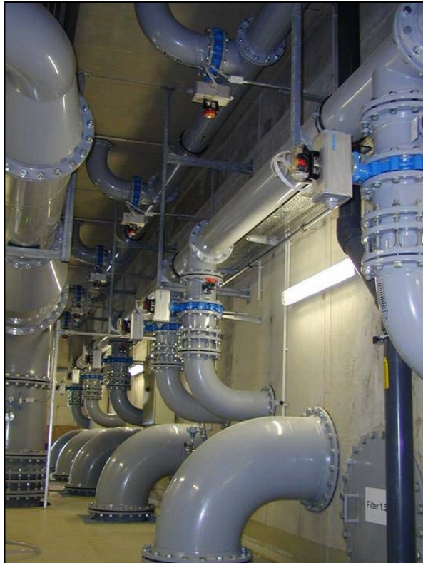
Figure 8: Pipe gallery in a water treatment system
