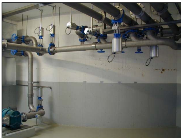
Figure 9: Pipe gallery in a wastewater treatment plant
