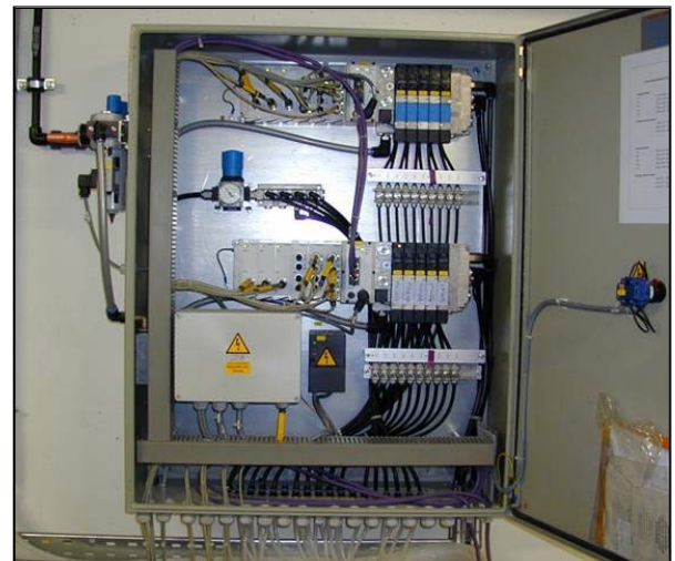
Figure 10: Control cabinet with valve terminal
