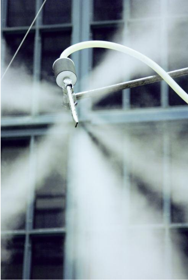
Steam leaving the diffusor. Condensation makes the steam visible.
