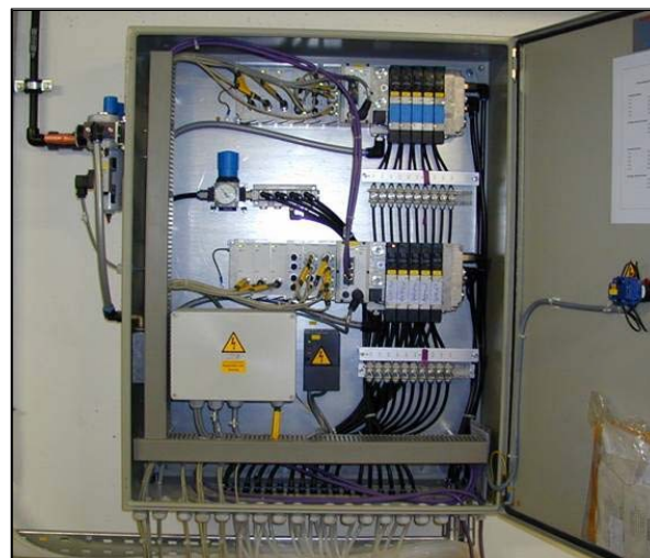
Figure 10: Control cabinet with valve terminal
