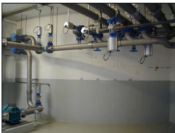
Figure 9: Pipe gallery in a wastewater treatment plant
