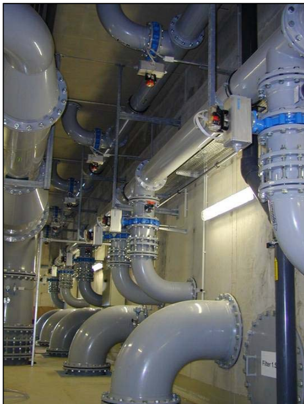
Figure 8: Pipe gallery in a water treatment system
